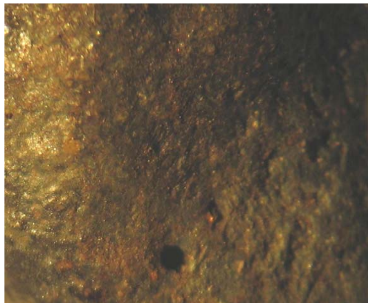
Brick burn material (exterior). Note smooth surface.
