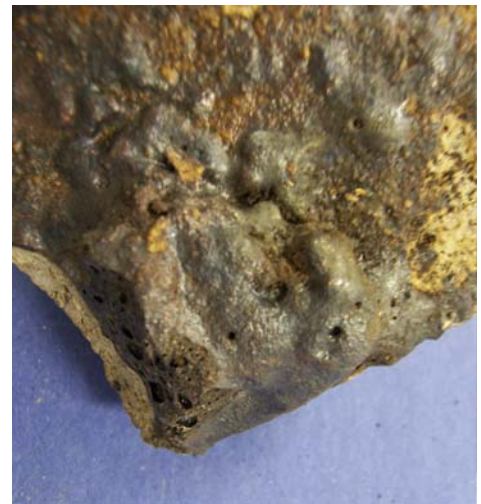
Brick—Burned area, closeup
